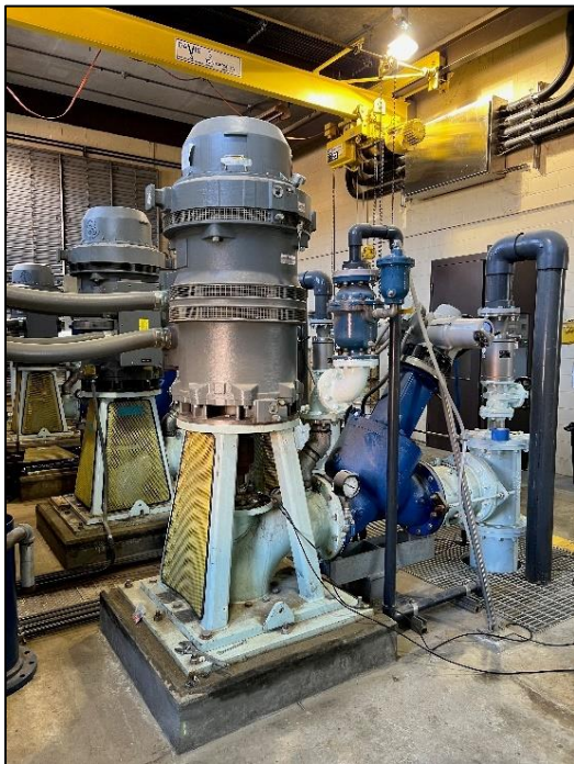
FIGURE 1: High Service Pump 1 at the JW Smith Pumping Station.
