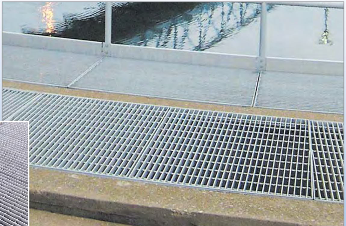
▲ LeMay WWTP - St. Louis, MO
