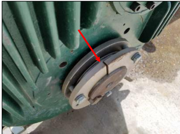
Figure C: Bushing Distortion due to Improper Key Installation.
